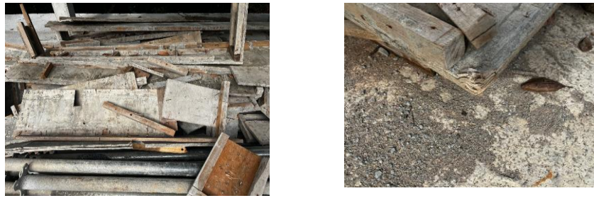
Figure 4: Damaged and discarded plywood formwork after reuse cycles
